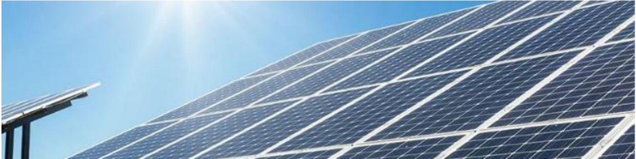
Figure 4-2 Rooftop PV system, for example only.
